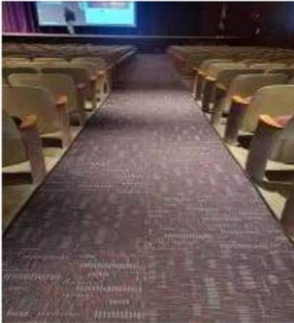
Photo #1 ACM black mastic beneath carpet (HA 02)
