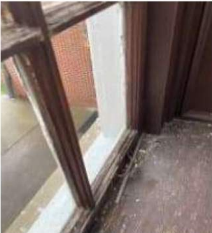
Photo #3 ACM interior window glazing (HA 03)
