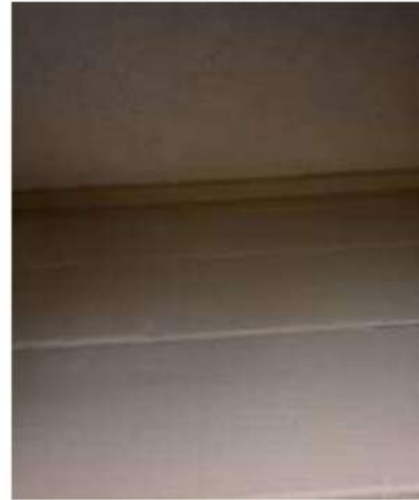
Photo #2 ACM filler material beneath paint on the concrete block walls (HA 01)
