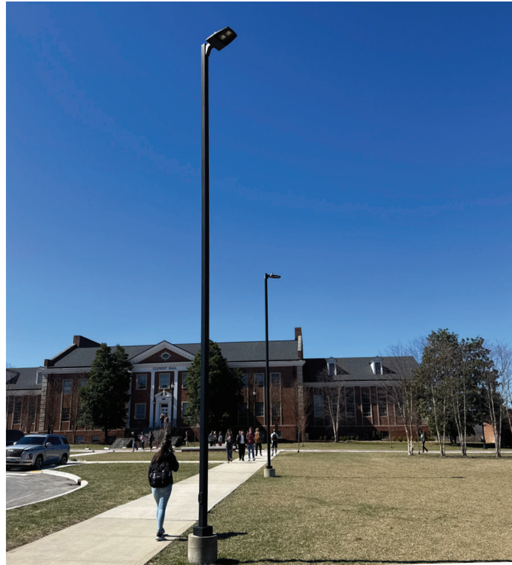
Typical Parking Area Light
